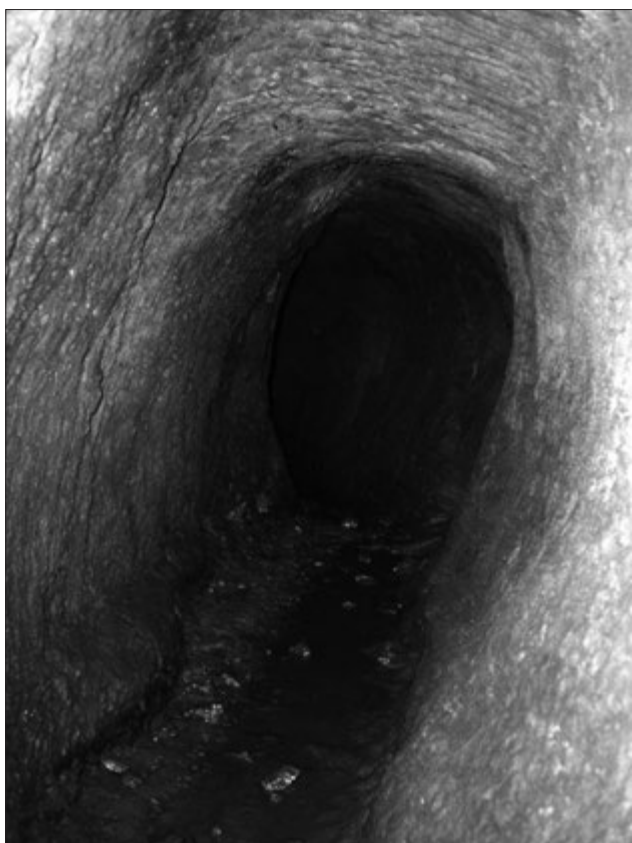
Fig. 13. Profile of the Venetian adit with ledge and channel (Photo M. Strassburger).
